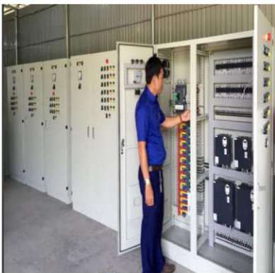
TỦ BOM DB PUMP
