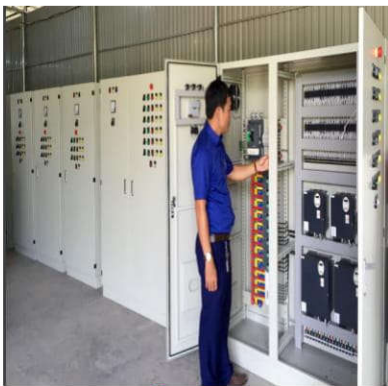
TỦ BOM DB PUMP
